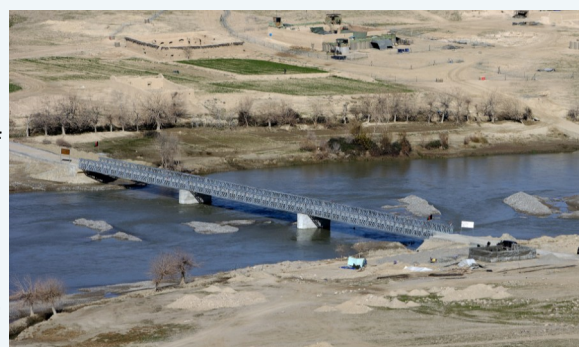
A bridge over the Helmand River, a project procured with NATO common funding using the CUR process.
